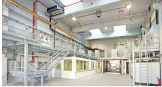
AIT Energy, Smart Electricity Systems and Technologies Laboratory, (SmartEST)
