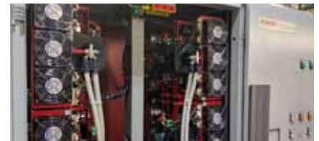
750 kVA inverter for testing of aircraft generators.
